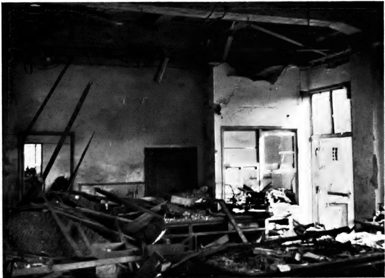
Photo No. 20. NAGASAKI. A room in the concrete hospital, \frac{1}{2} mile from the centre of damage. The building was structurally undamaged, and one of the few of its type to escape internal fire damage. The collapse of suspended ceilings, partitions, etc., caused many casualties; fire would have increased their plight. See paragraphs 68 and 80.
